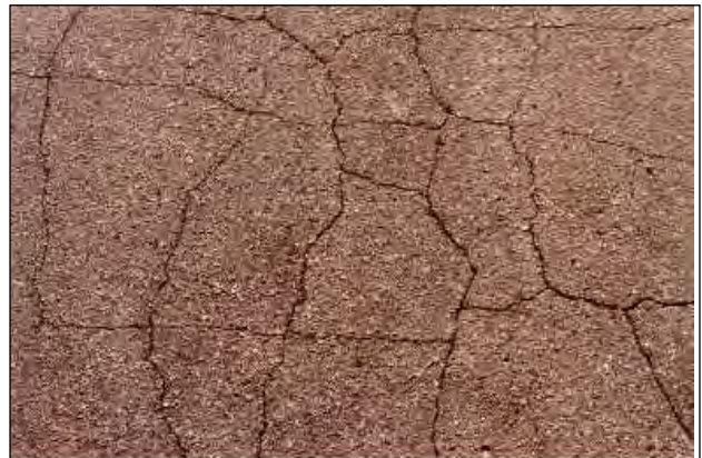
Condition 5 – Very Poor
